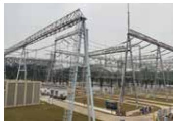
Electricity power inspection
